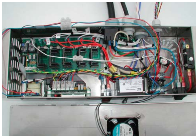
3 Gp Electrical Box, Nov 2004
